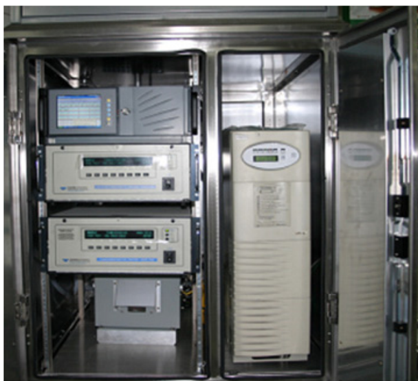
Fig. 5. Telemonitoring system (TMS) at B-subway station used in this study.
