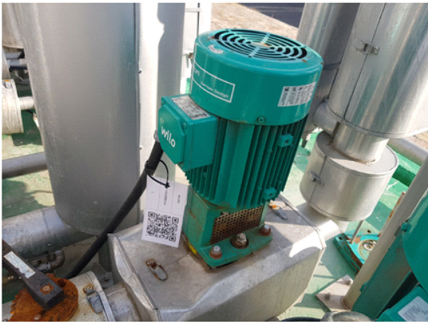
Fig. 10. Equipment with a QR code attached.
