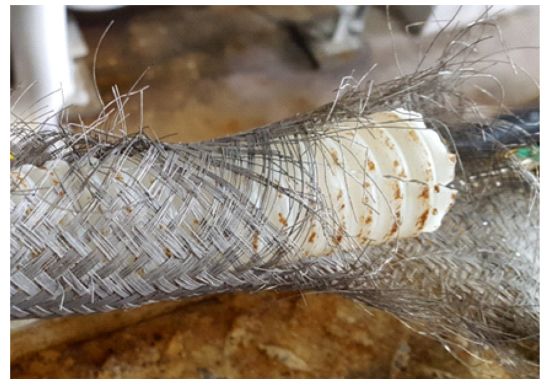
Fig. 7. Corroded flexible hose.
